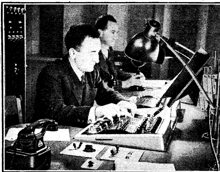
MODERNISING THE D.C. PANEL. Two new dramatic control panels which have just been installed in Berlin Broadcasting House. The sliding controls greatly facilitate the handling of multiple studio outputs by one man. Economy of space is another great advantage.
